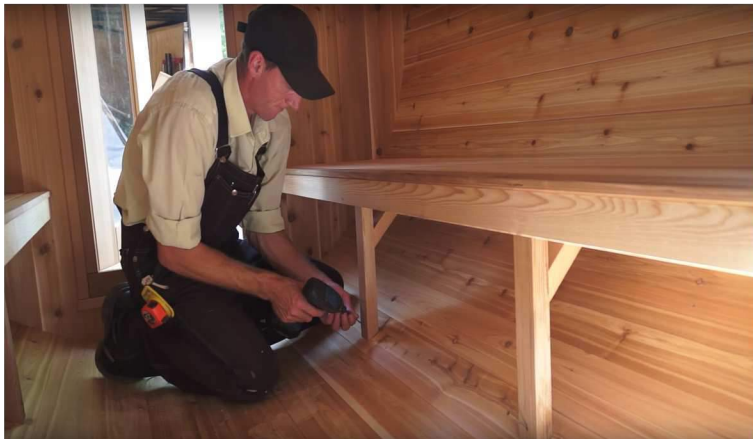
35. Screw bench supports into floor with 2 1/2" screws. Repeat above steps for other bench.
