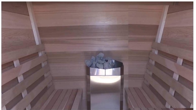
EH-6. Space rocks out evenly in top of heater.
