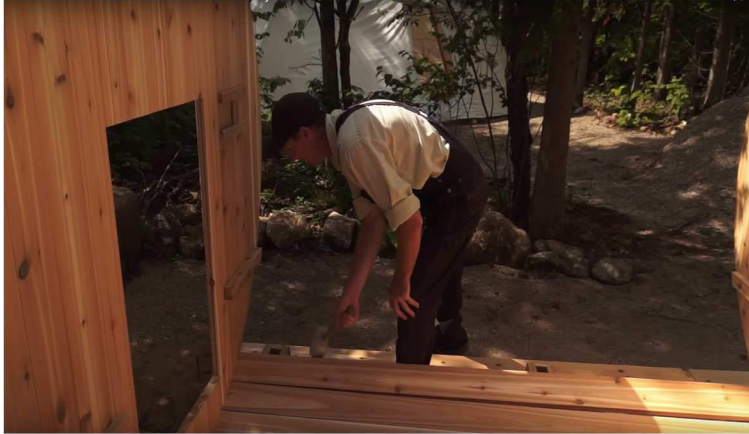
15. Use the rubber mallet to tap wall staves tight to each other.
