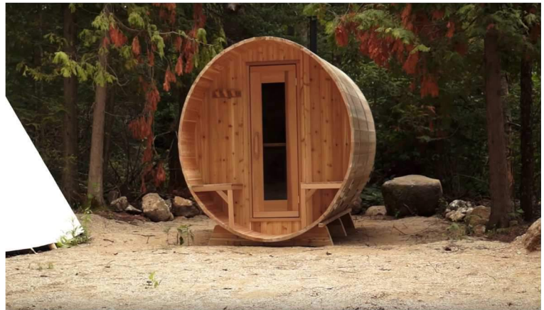
44. Repeat on other porch seat ensuring they are level with each other.
