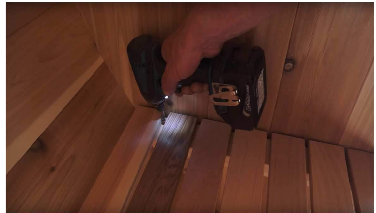
32. Secure benches to wall supports by attaching with 1 1/2" screws in between bench slats.
