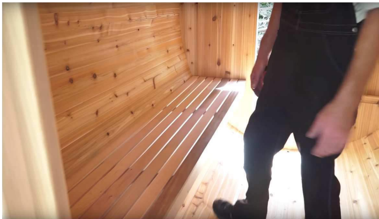
31. Place the long benches down on the wall brackets and then snug up against the back wall.
